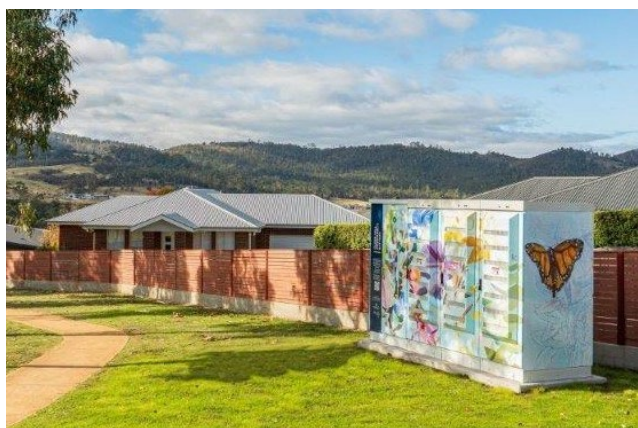
Figure 1: Glebe Hill Community Battery
