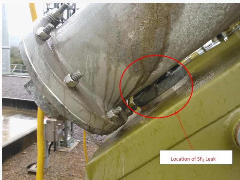
Figure 6: Persistent SF6 leak on switchgear
