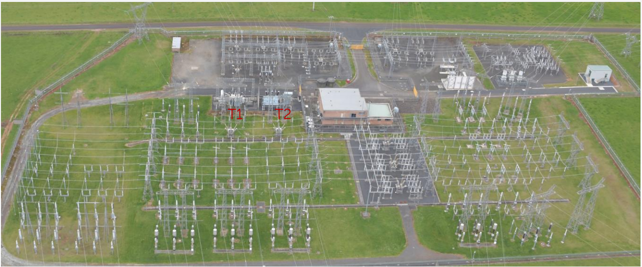
Figure 5: Aerial view of Sheffield Substation
