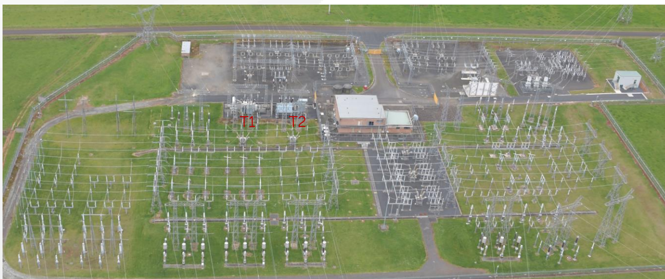
Figure 6: Aerial view of Sheffield Substation
