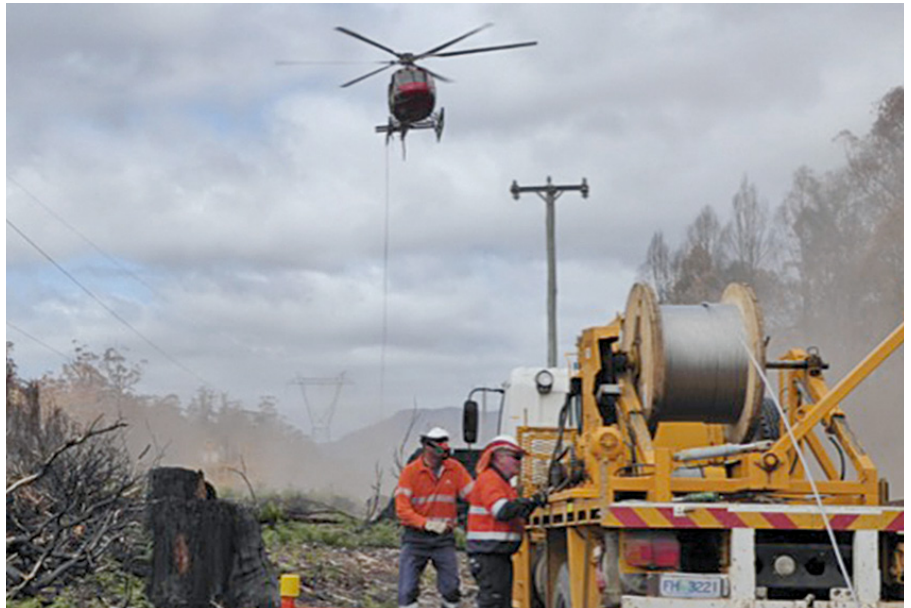
Airborne sediment generated from construction activities can cause localised air pollution and become a safety risk
