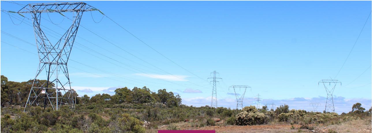
The Waddamana to Palmerston transmission lines are critical for energy security in Tasmania.
