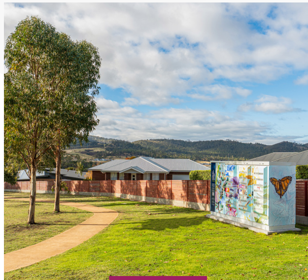
The community battery is up and running in Glebe Hill.
